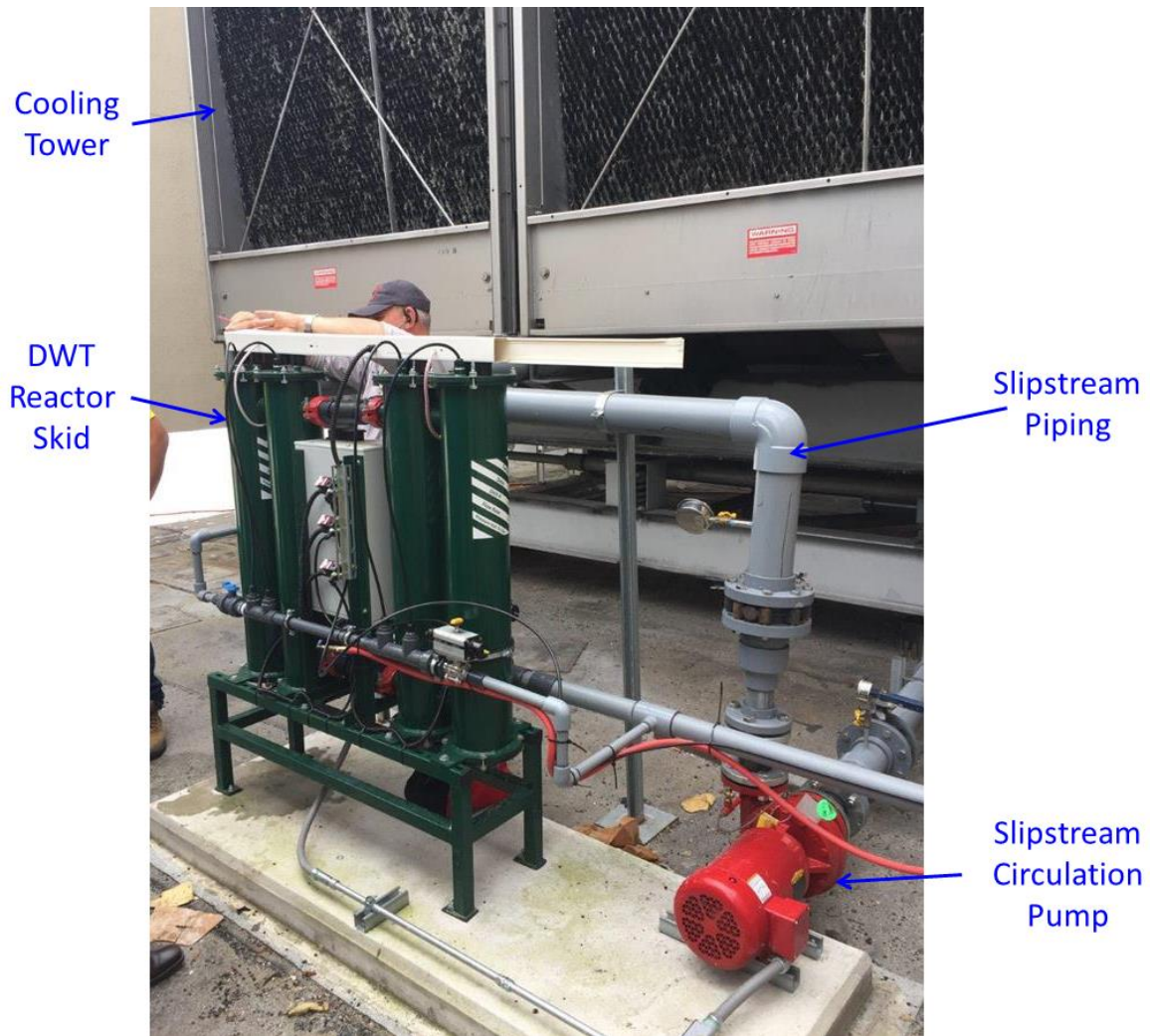
Figure 3. AWT System and Associated Piping and Pumping (Credit: Gregg Tomberlin, NREL)
